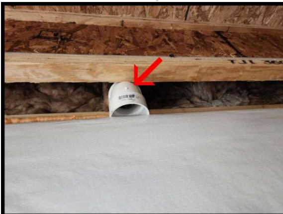
Waste drain lines.
