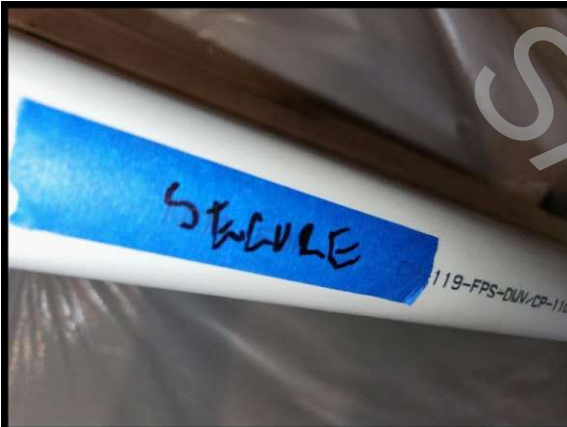
Sump pump discharge.
