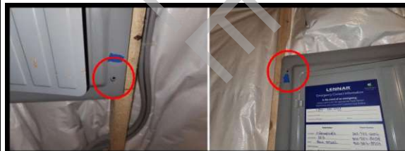
Main electrical panel.
