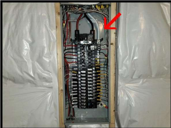
Main electrical panel.
