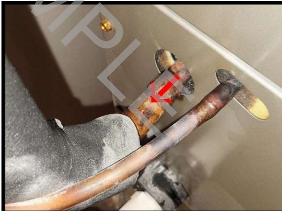
HVAC line set.
