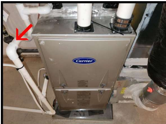
Condensate drain line.
