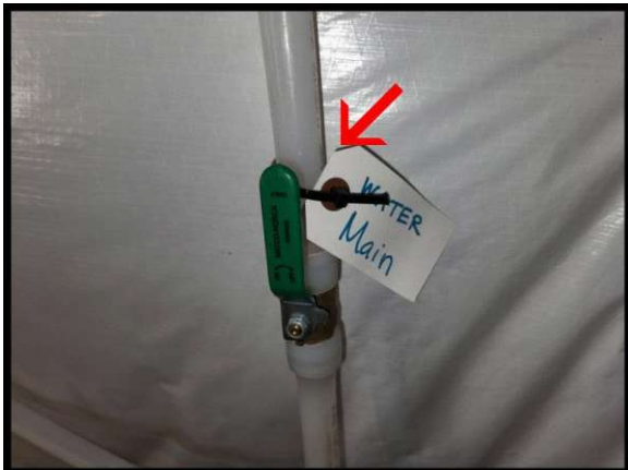
Main water shutoff valve.
