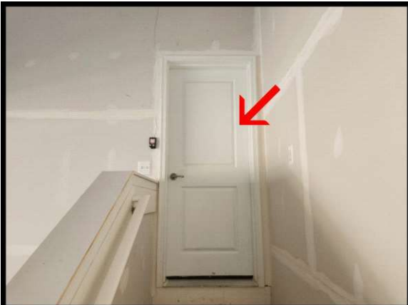
Garage fire door.
