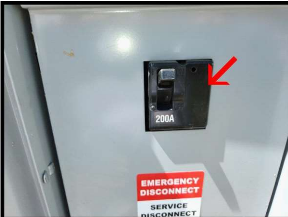
Exterior service disconnect switch.
