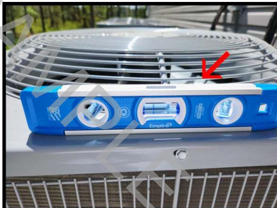
Outdoor condensing unit.
